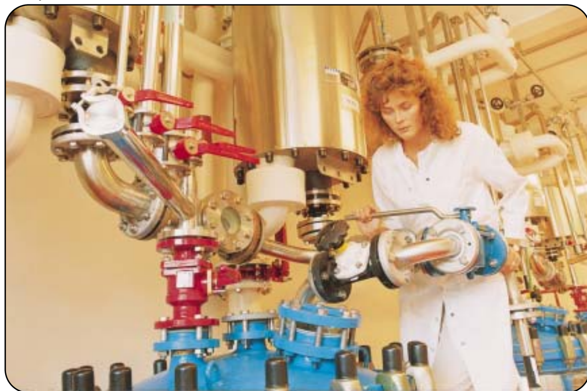
Vent piping for pharmaceutical manufacturing in 654 SMO®
