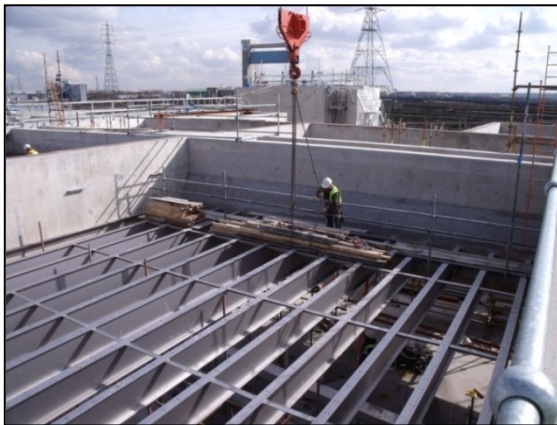
Fig. 5 Stainless steel I-shaped beams at Thames Gateway Water Treatment Works Photo: Interserve
