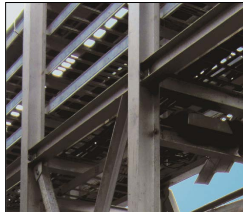
Fig. 2 Stainless steel frame in nuclear power plant
